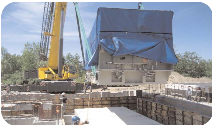
Brookfield, CT: Positioning the compressor unit onto its foundation within the station building.
