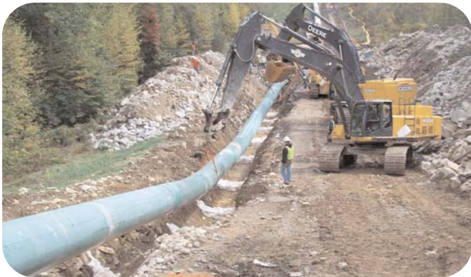
Newtown, CT: A section of the pipeline loop is placed in ditch.
