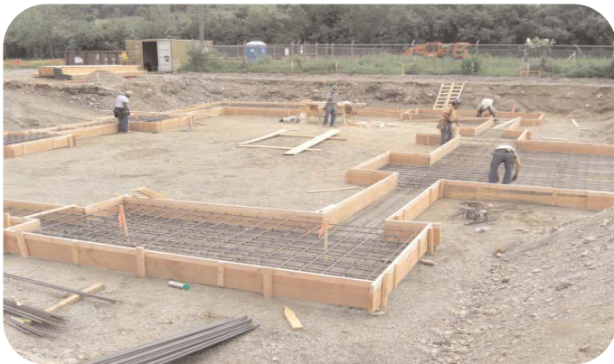
Milford, CT: Laying out the foundation forms for the new compressor station.
