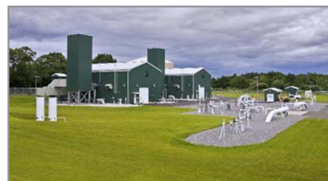
Phase II: Two compressor units placed in service at Milford Compressor Station
